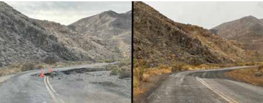
Emigrant Canyon at milepost 5.1 before & after repair. Federal Highway Administration
